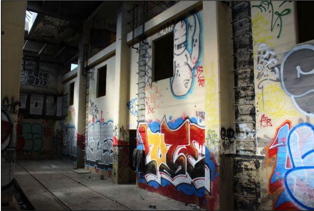
Photograph 15: Main control floor with rail line through the center, camera facing southwest. April 29, 2021.
