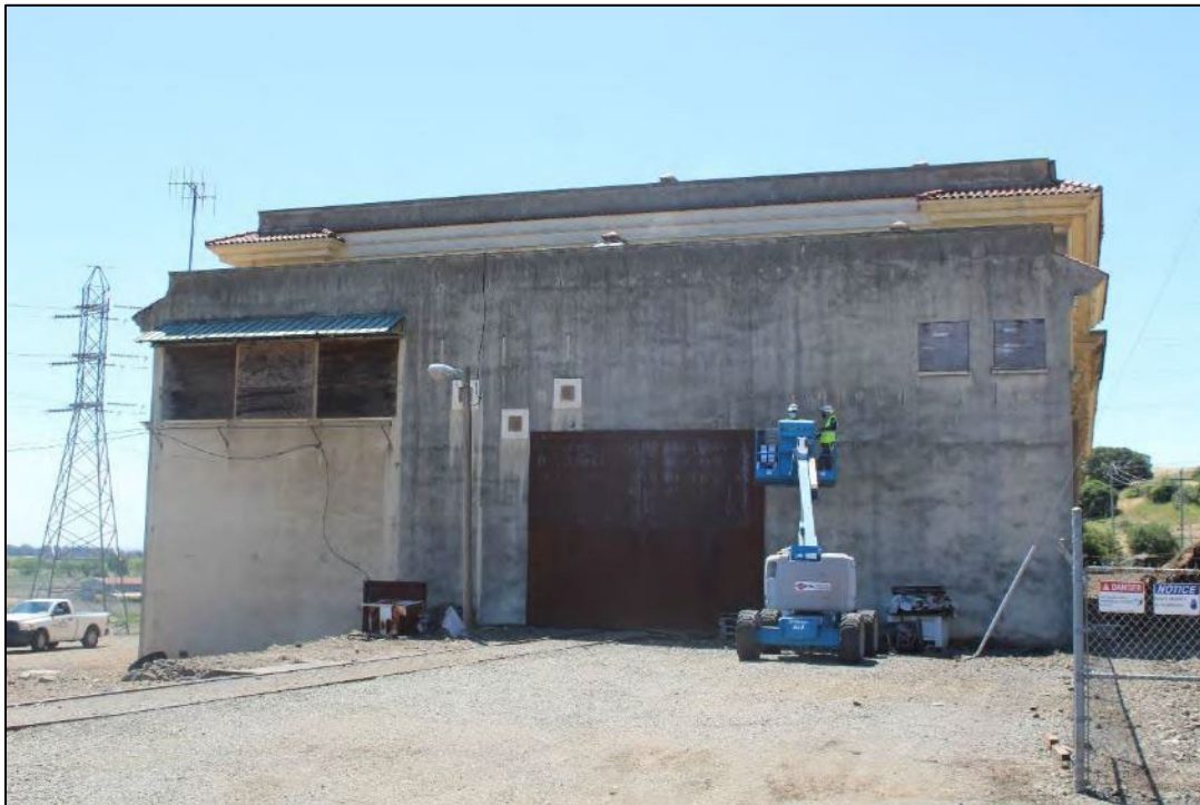
Photograph 4: Kinnear door covered by steel plate on the north elevation, camera facing southeast. April 29, 2021.
