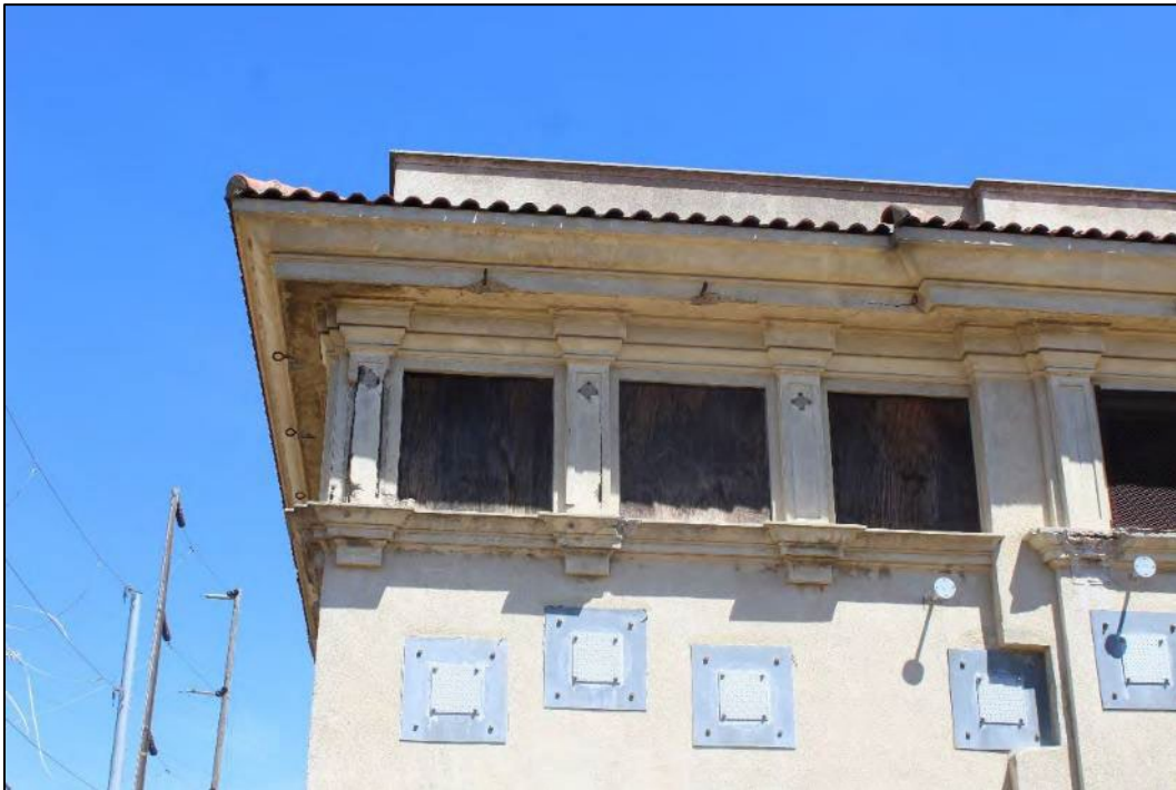
Photograph 12: Visible spalling of concrete cornice and pilasters on the south elevation, camera facing north. April 29, 2021.
