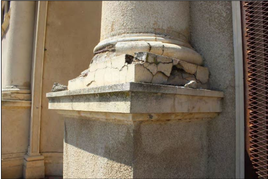
Photograph 7: Cracking and spalling of concrete columns, camera facing southwest. April 29, 2021.
