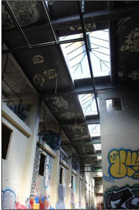
Photograph 16: Ceiling spalling inside the control building, camera facing southeast. April 29, 2021.
