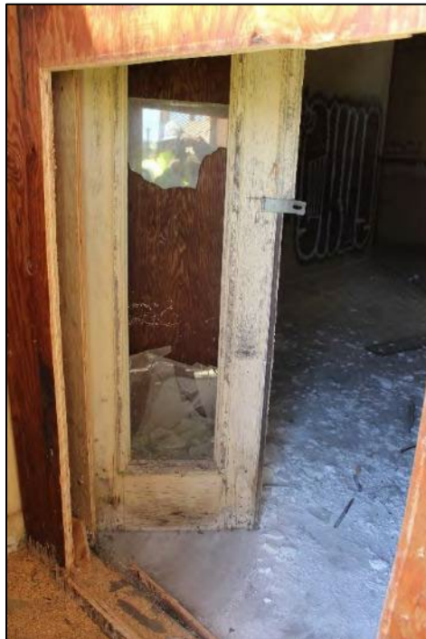
Photograph 8: Glazed doors with broken glass, camera facing southwest. April 29, 2021.
