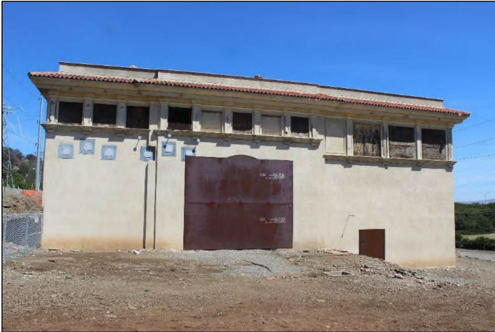
Photograph 3: Kinnear door covered by steel plate on the south elevation, camera facing north. April 29, 2021.
